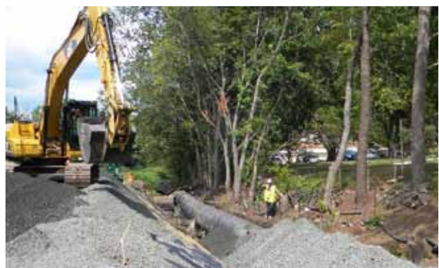
Installation of bypass piping to manage the flow of Coles Brook during soil remediation at the 111 Essex Street, Maywood property.
